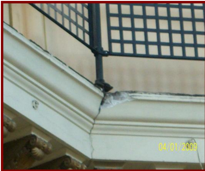
Above: A portion of the cracked and missing plaster below where the catwalk railing is attached.
